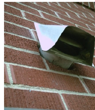
Dryer vent stuck open – Clean and seal with steel wool.
